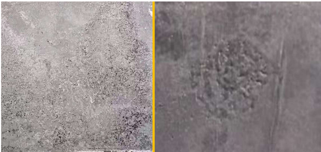
FG 18: Surface carbon defect by burning before pouring process.
